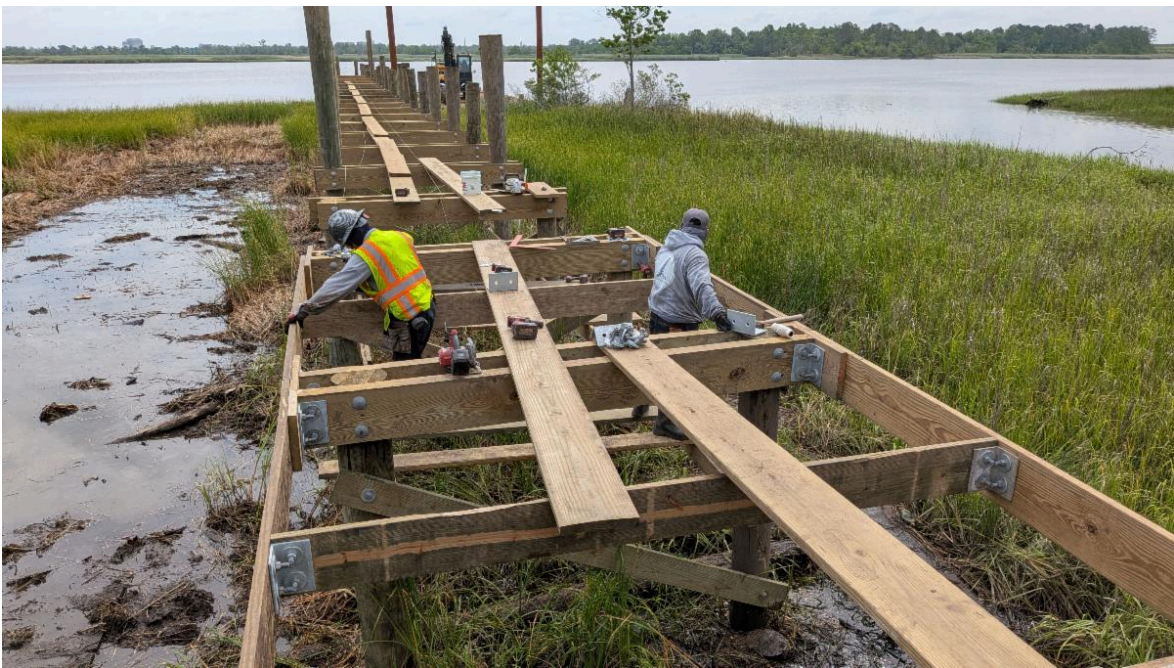
Decking platforms are still being constructed near the water. Work is going quickly for the TD Eure crew.
