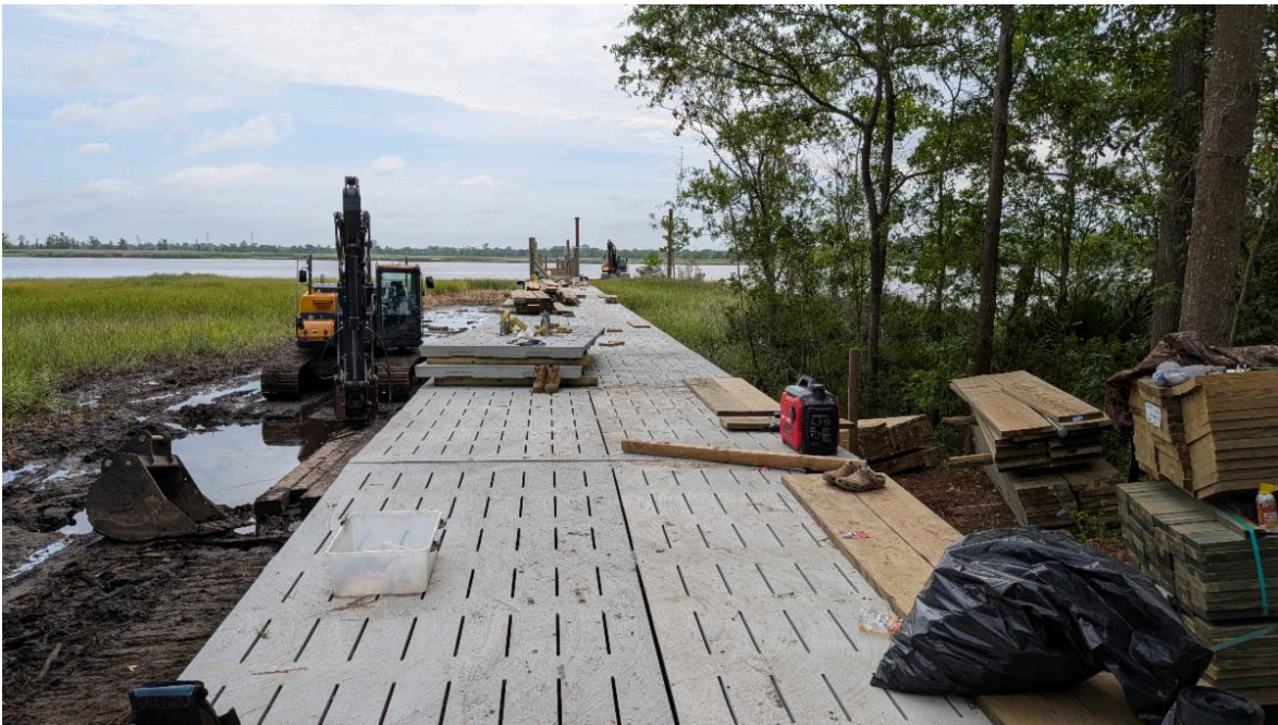
Looking toward the Brunswick River, the boardwalk extension is laid in 5 foot sections (the boardwalk is 10 feet wide). The concrete decking is then mounted to pylons and railings. Much thanks to our marine contractor, TD Eure.
